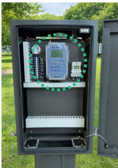
Controller in distribution board
