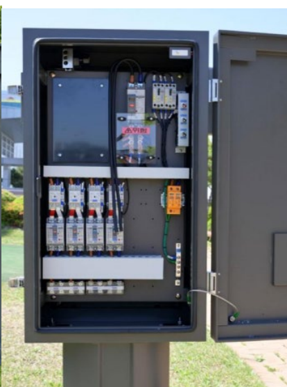
4 channel distribution board
