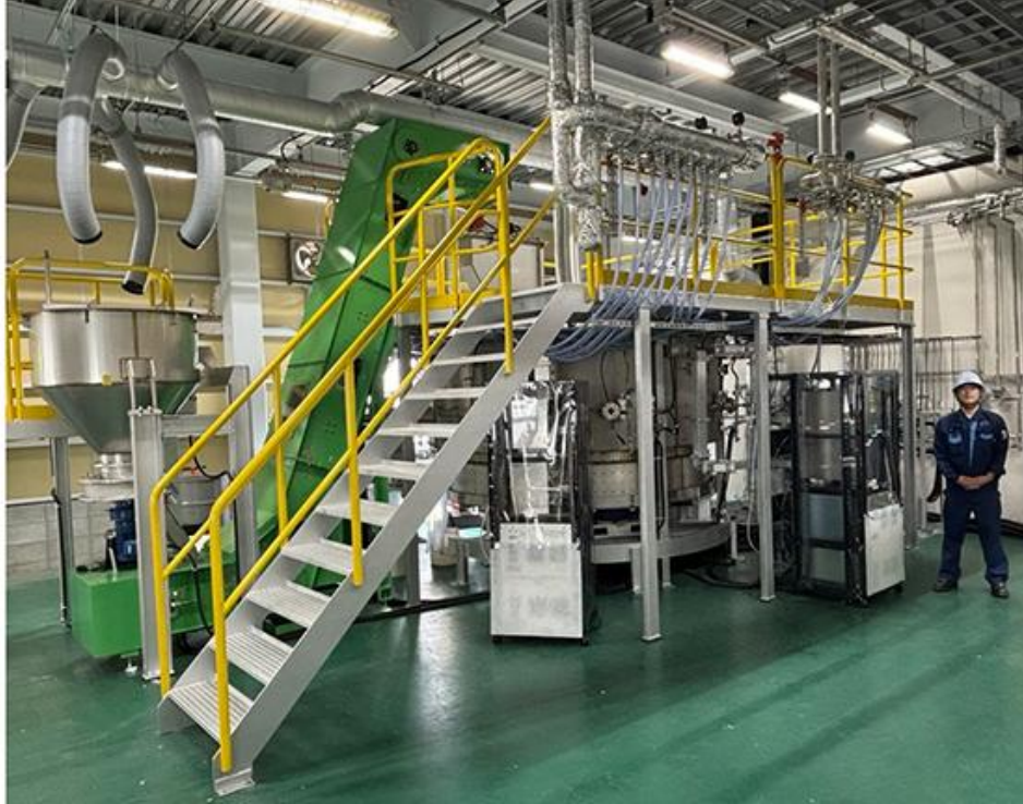
Figure 1: MWCC – Mitsui Pilot Plant, Osaka
