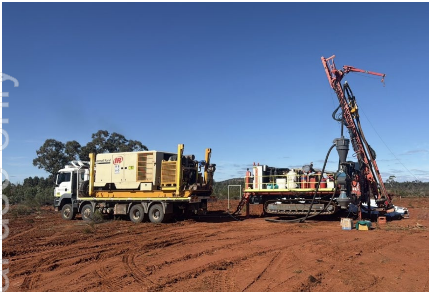
Photo of the Dual purpose, track mounted rig that will shortly be mobilised to the Horn Island gold project.
