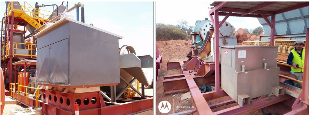
Figure 11: Ball Mill frame, motor and Liquid resistance Starter
