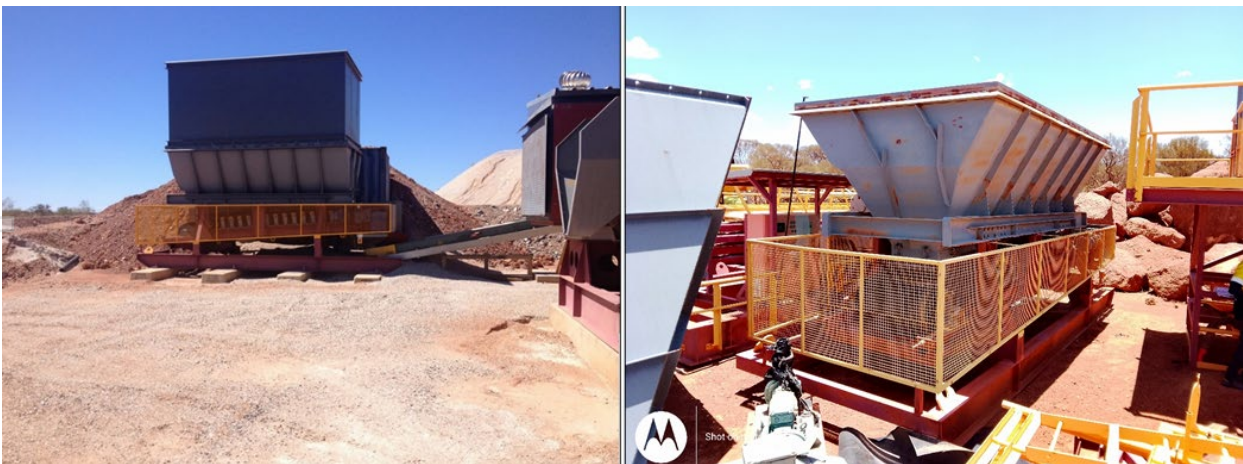
Figure 3: ROM Bin Components
