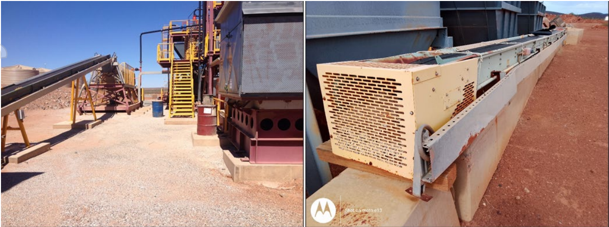
Figure 4: Rom Bin to Mill conveyor
