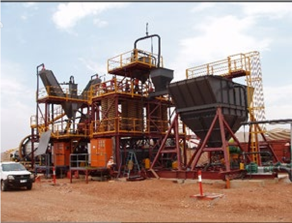
Figure 2: Modular Gravity Plant Installed and operational (as previously operated)
