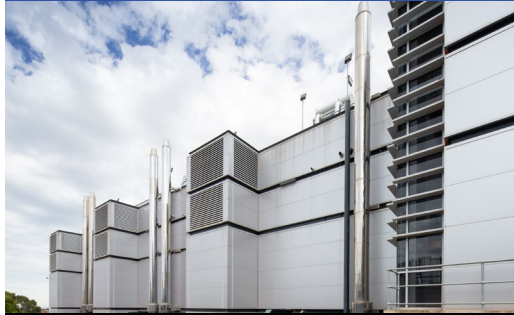
TELSTRA DATA CENTRE, CLAYTON VIC
