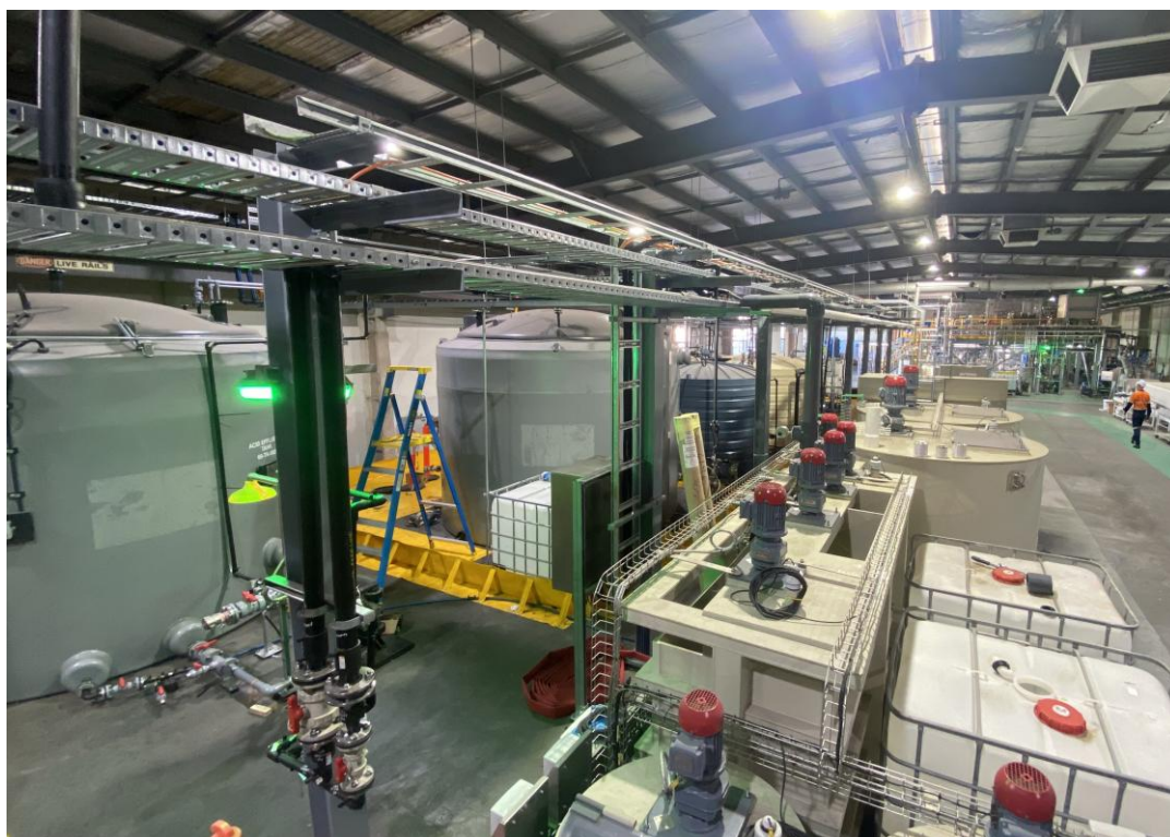
Figure 1. Renascor's PSG Demonstration Facility
