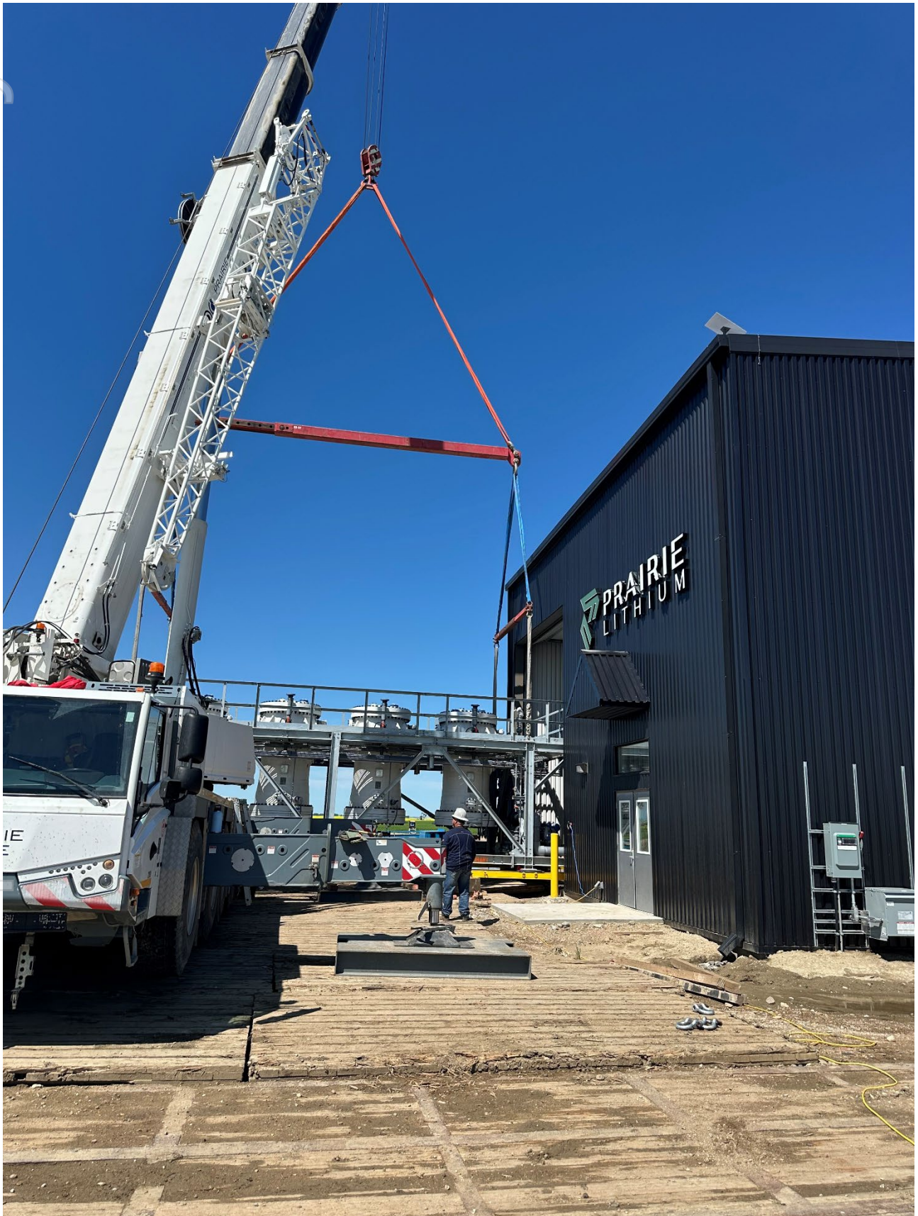
Figure 2: Prairie Lithium's four-column Commercial Scale DLE Unit at Prairie Lithium site
