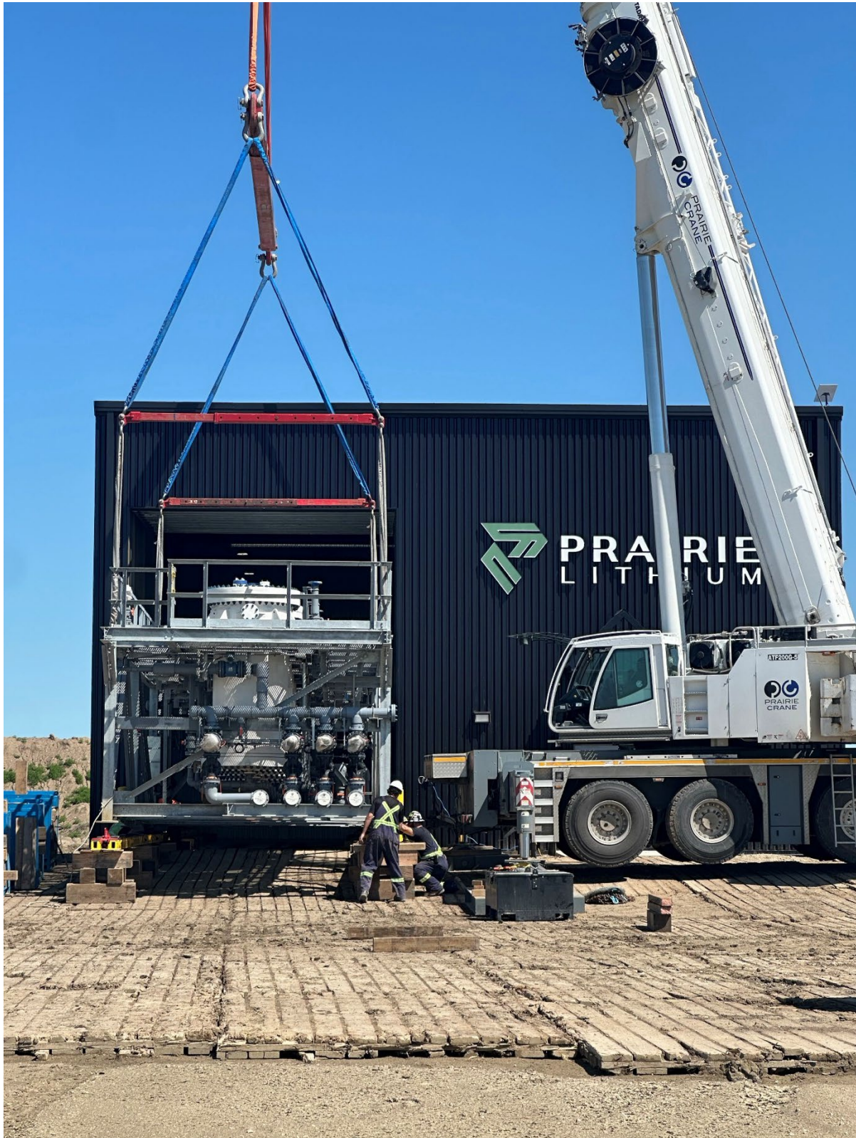
Figure 1: Prairie Lithium's four-column Commercial Scale DLE Unit at Prairie Lithium site
