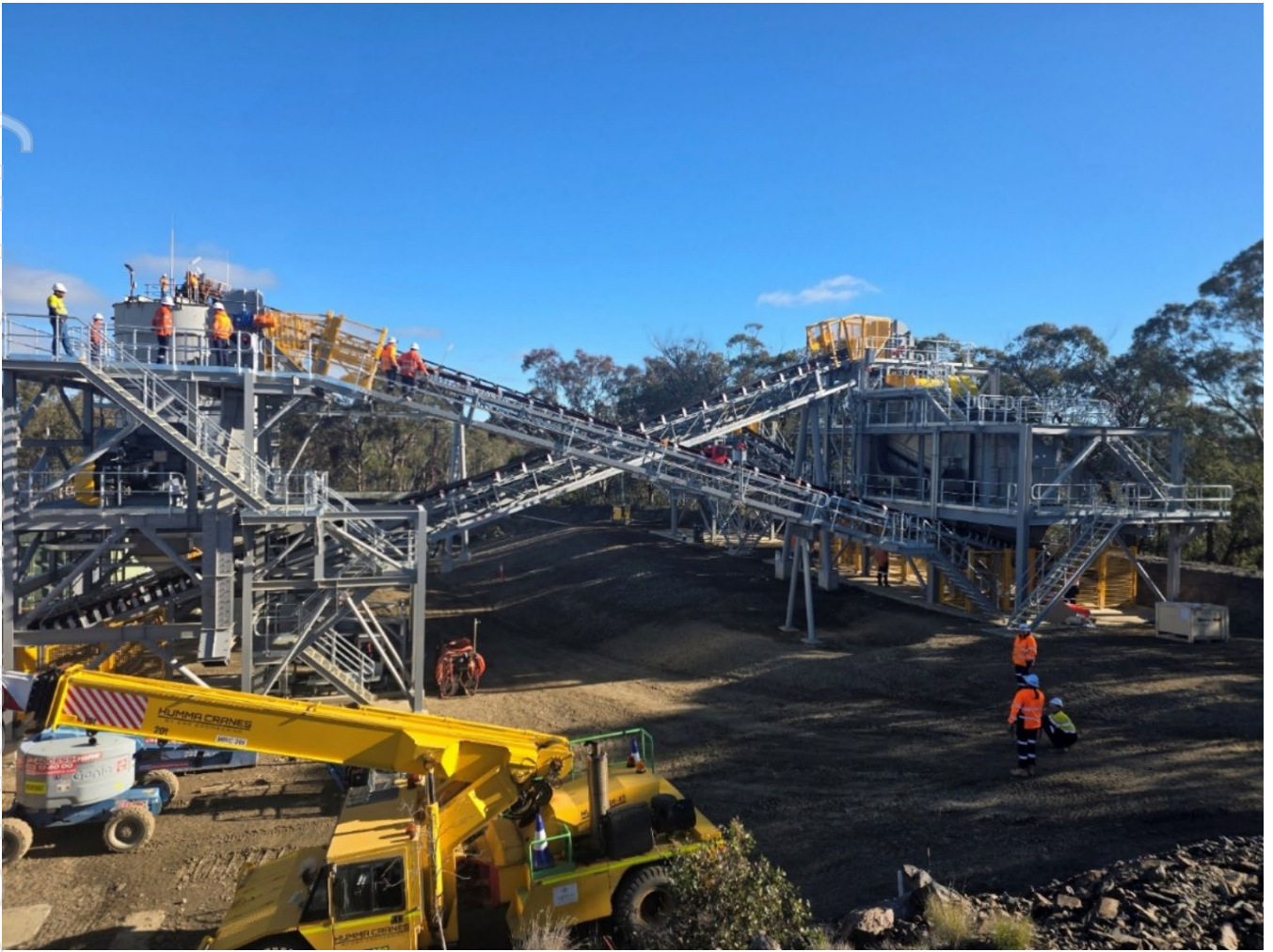
Figure 3 Closed circuit secondary crusher (left) and screen deck (right)
