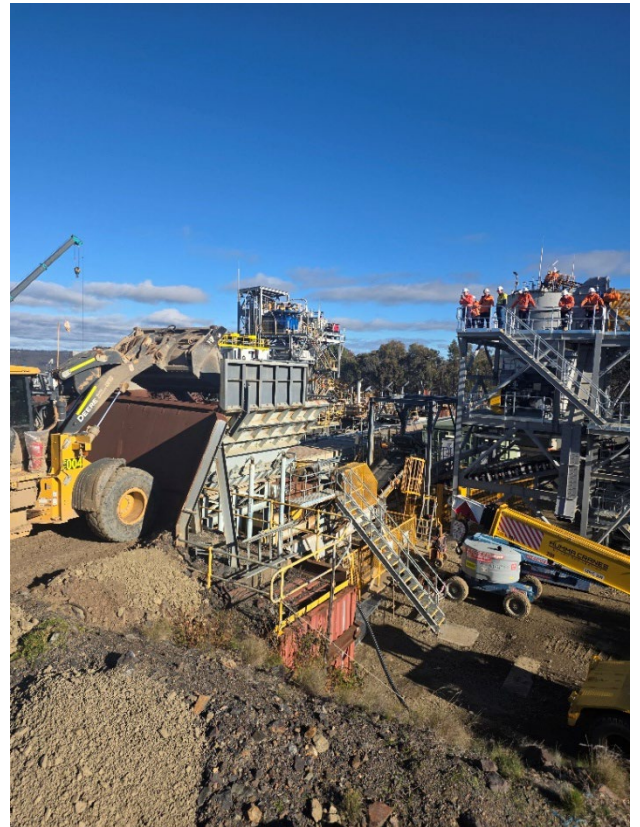
Figure 2 First ore into Jaw crusher hopper, Secondary crusher on right
