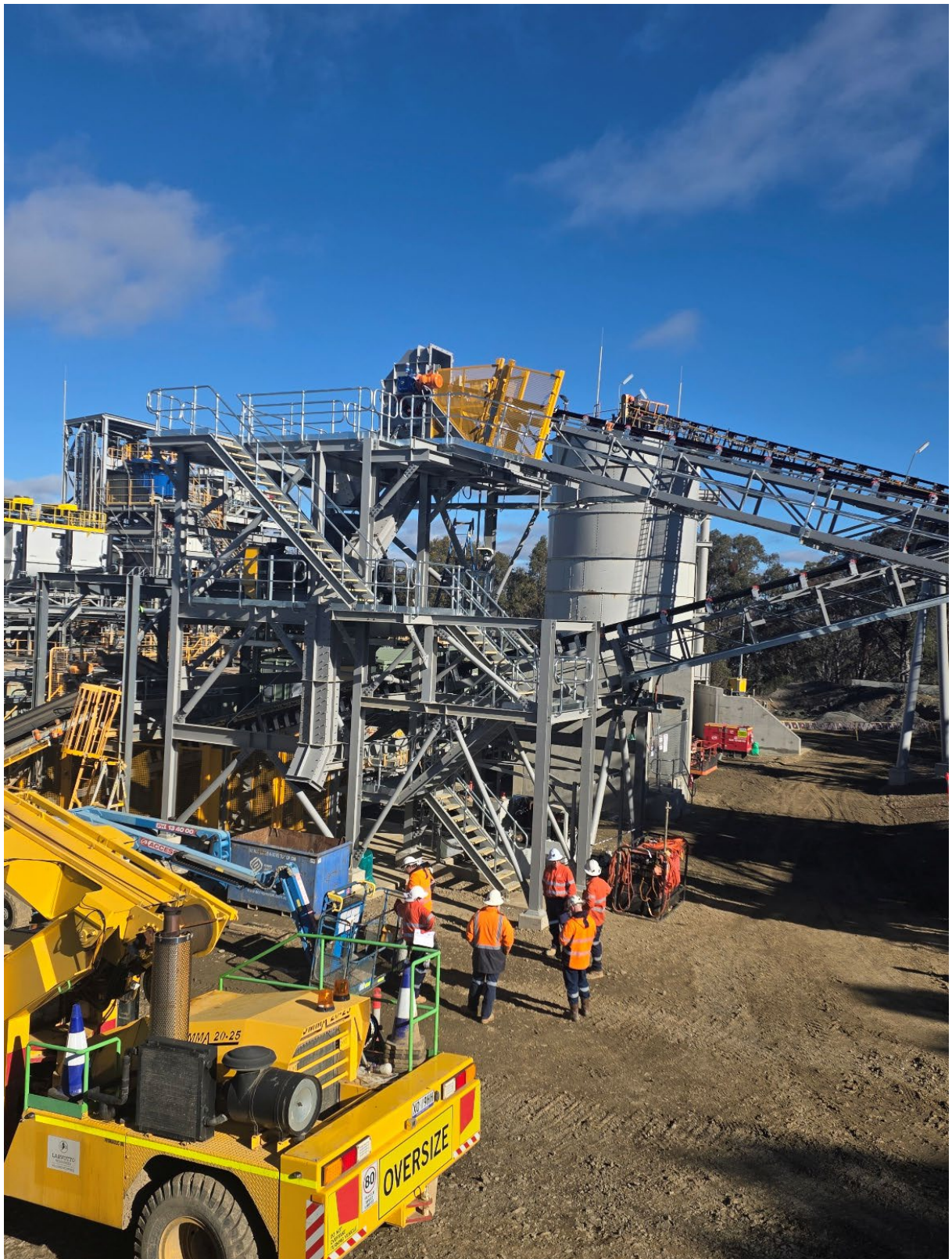
Figure 4 Secondary crusher with fine ore bin at rear
