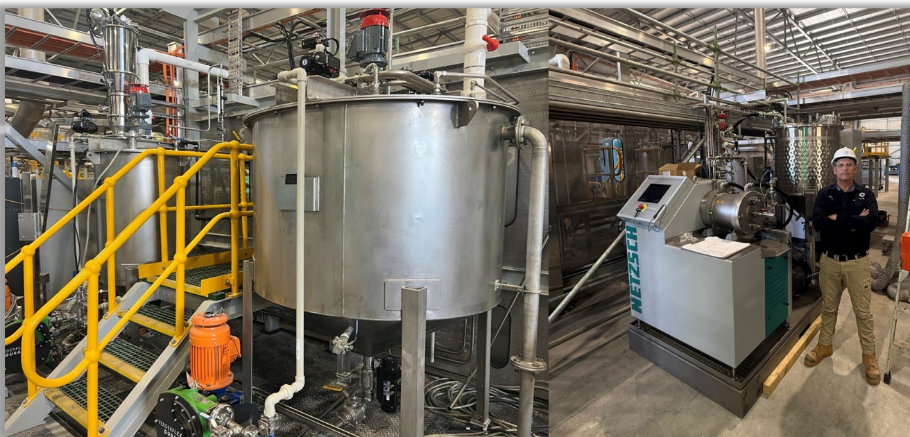
Installed HPA nano-mill and supporting equipment
