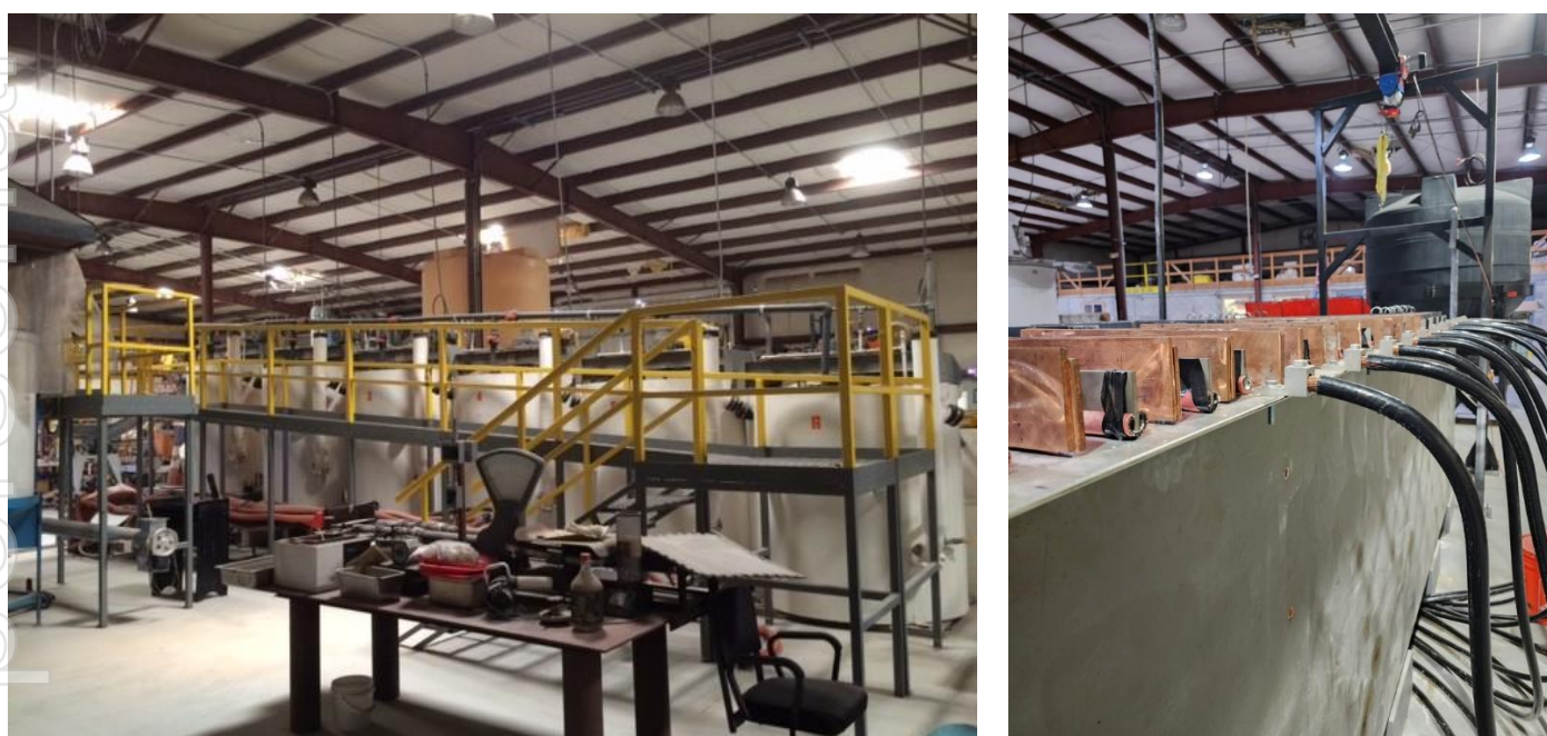
Figure 3 & 4: Infrastructure at the Del Sol facility
