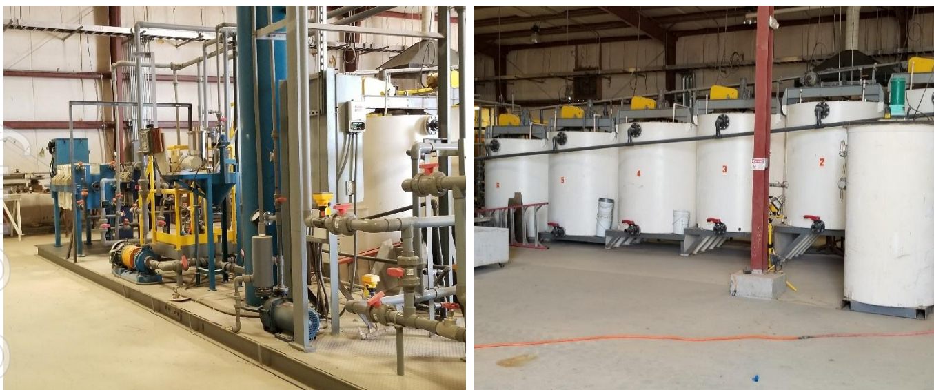
Figure 1 & 2: Infrastructure at the Del Sol facility
