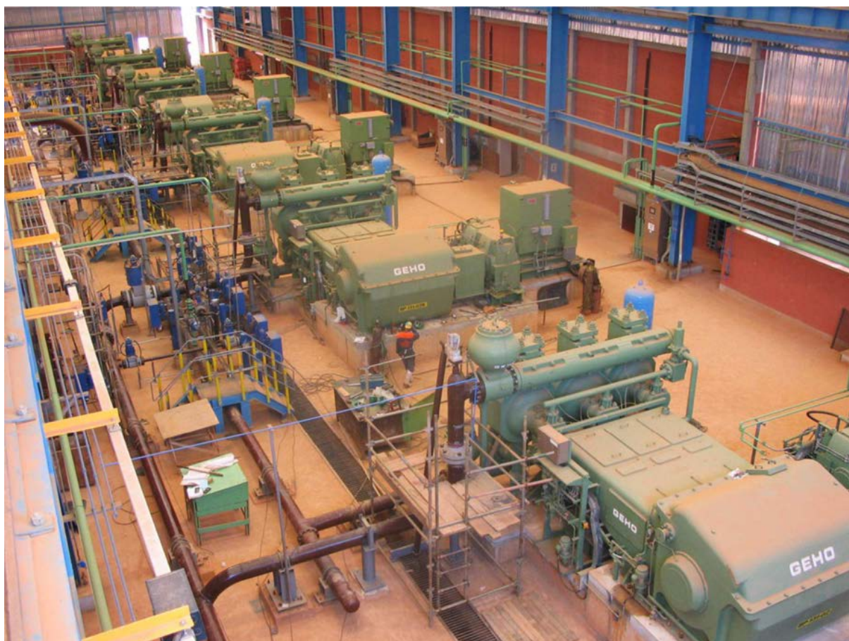
Figure 22: Reference site slurry pump house. Courtesy Fortin Pipelines.
