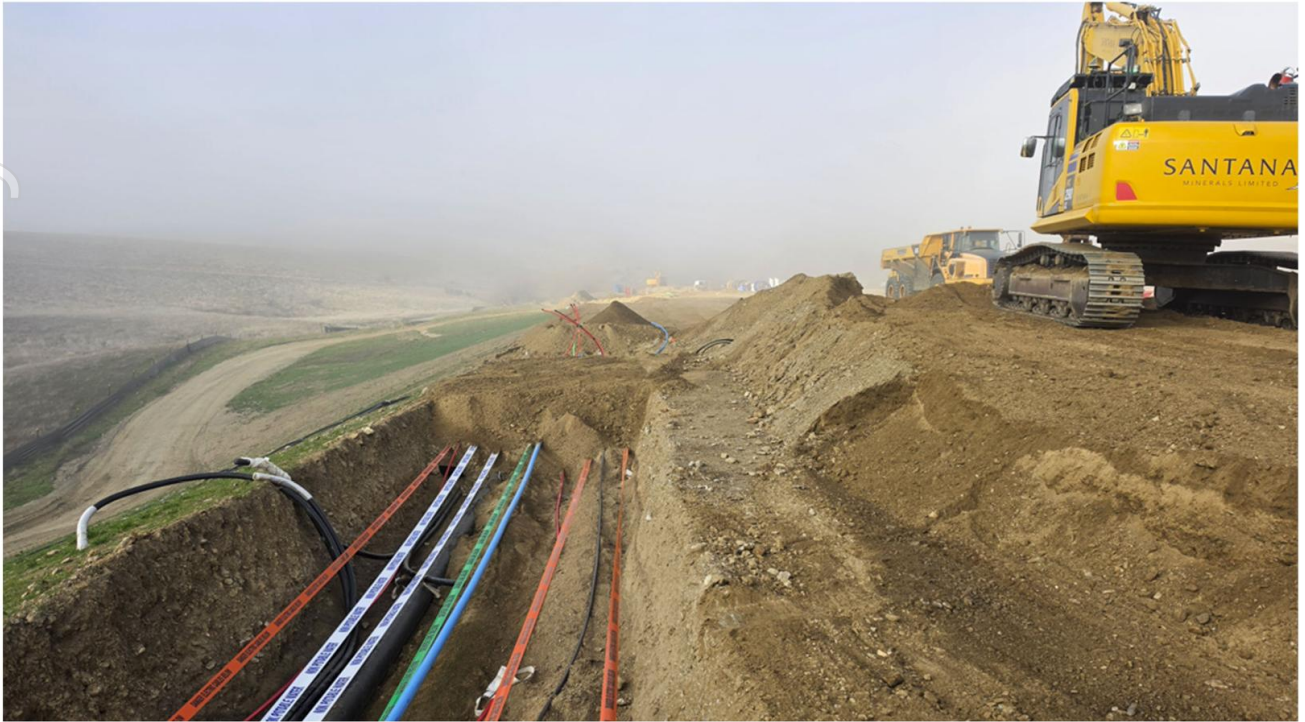
Figure 3. Common services trench on Ardgour Station: HV-LV power, sewerage, potable water and communications
