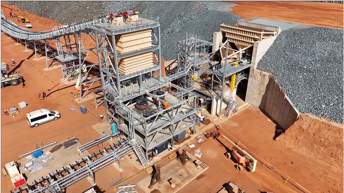
Karlawinda Expansion Project – Primary/Secondary/Tertiary crusher building and ROM 2.
