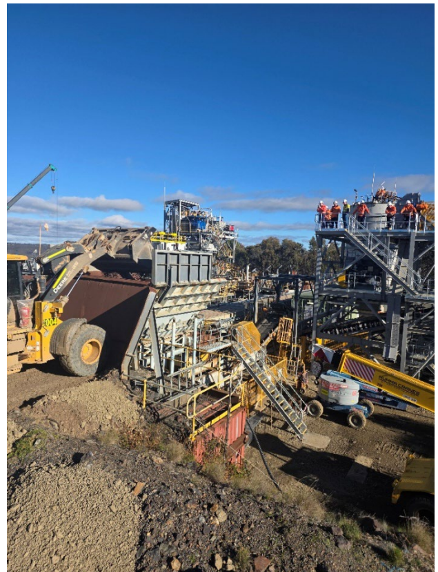
Figure 3 First ore into jaw crusher hopper, secondary crusher on right
