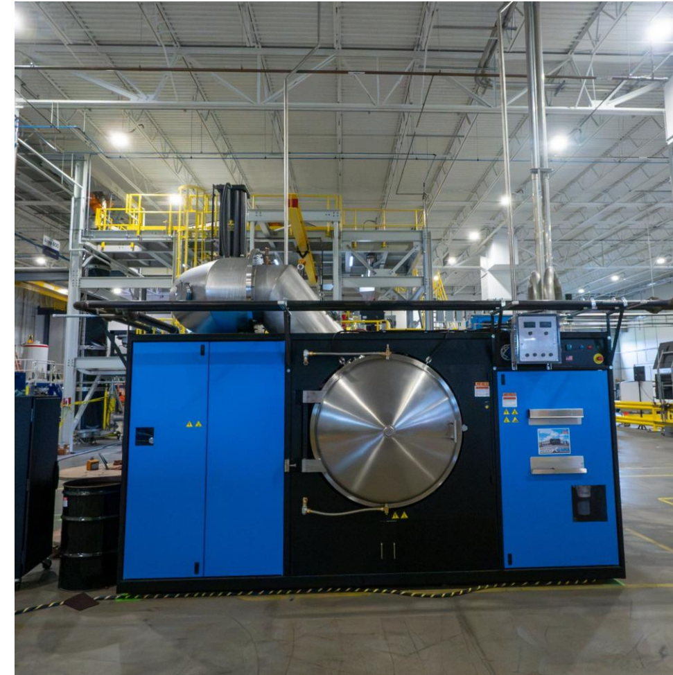
New sintering furnace delivered and being commissioned
