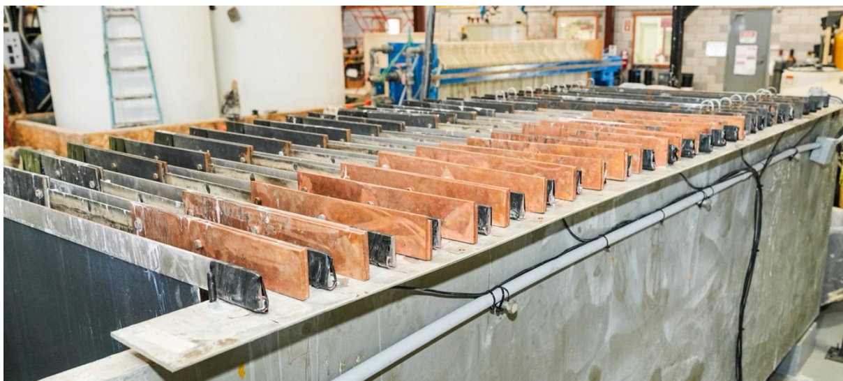
Figure 4: Internal view of the Del Sol processing building, showing electrowinning cells.
