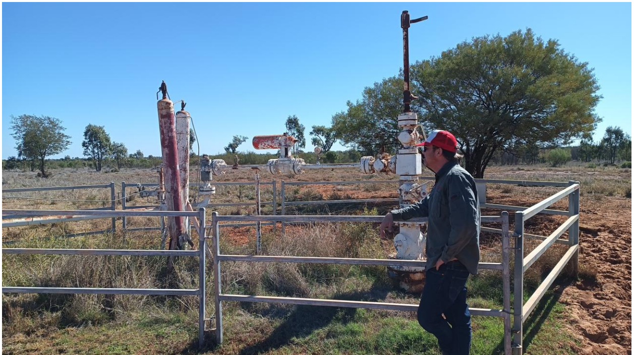
Figure 7 Major-4 with pressure gauges and defoamers inspected ahead of formalising timeline for production of Major gas
