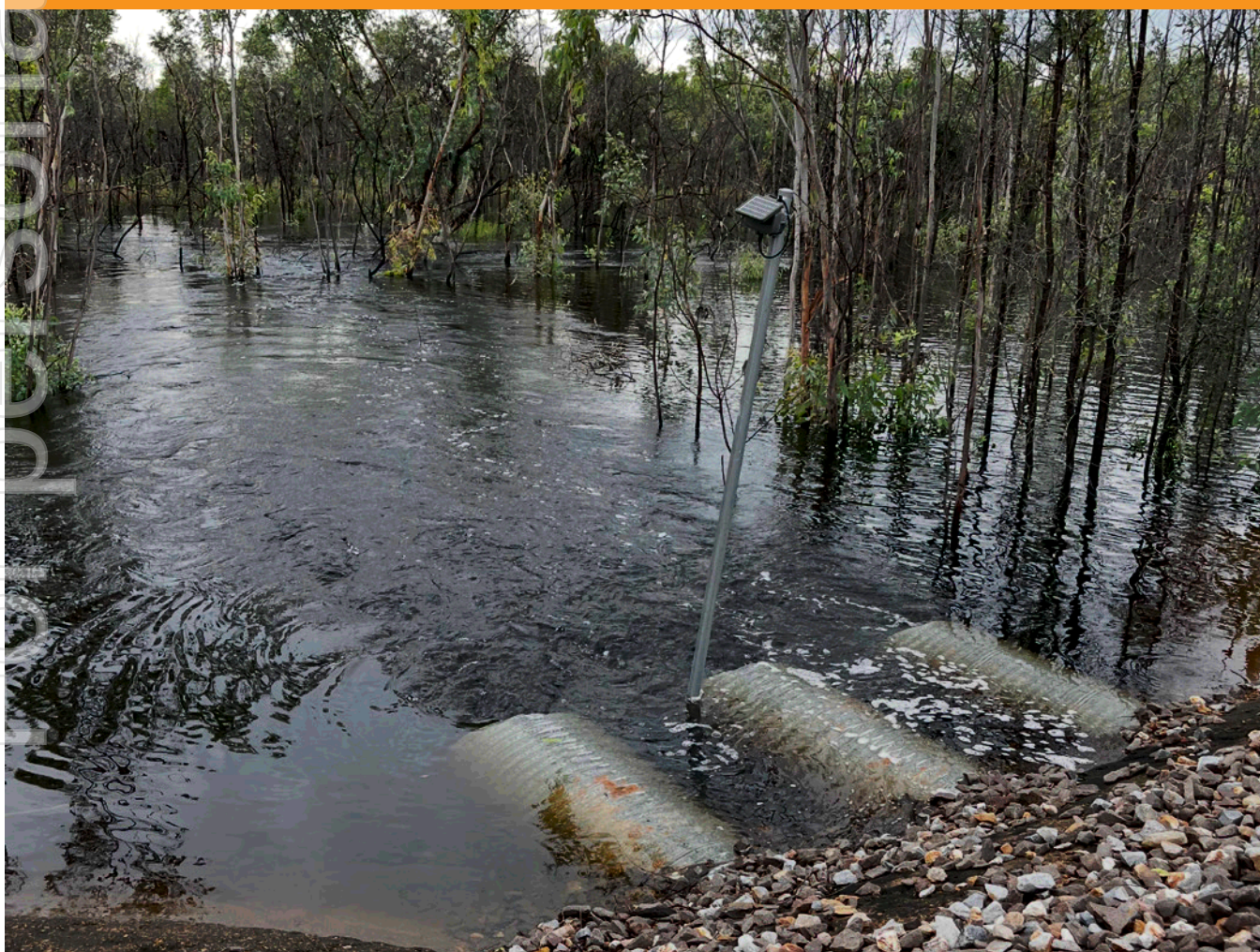
Floodwaters impacting rail infrastructure along the Taroocola to Darwin rail network.
