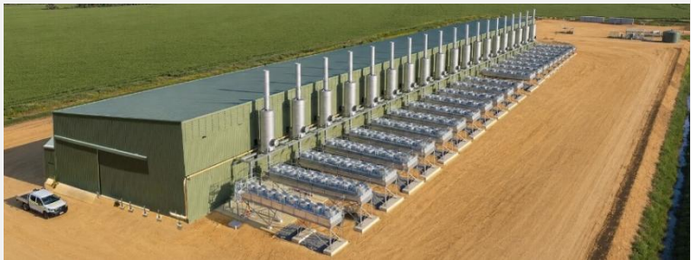
85MW WA power station
