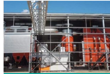
Biomass Steam & Hot Water Generation
