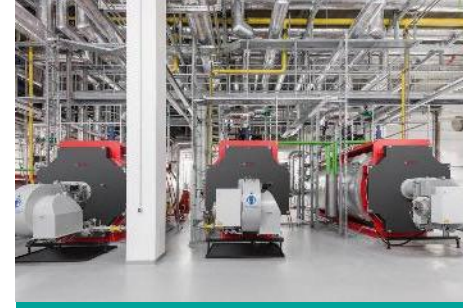
Industrial Package Boiler
