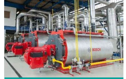
Large Commercial Hot Water Boilers
