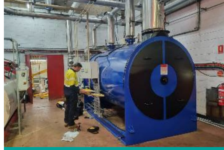
Industrial Steam Boiler
