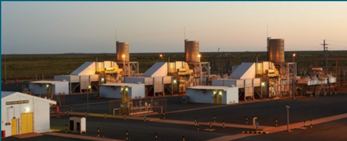
Image: Port Hedland Power Station, WA
