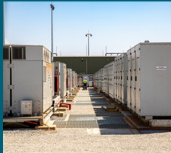
Image: Port Hedland BESS, WA
