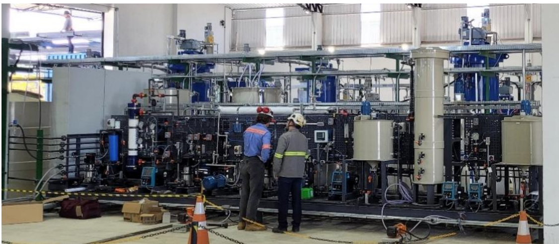
Figure 16: Water Treatment and Recovery Package at MREC Demonstration Plant.
