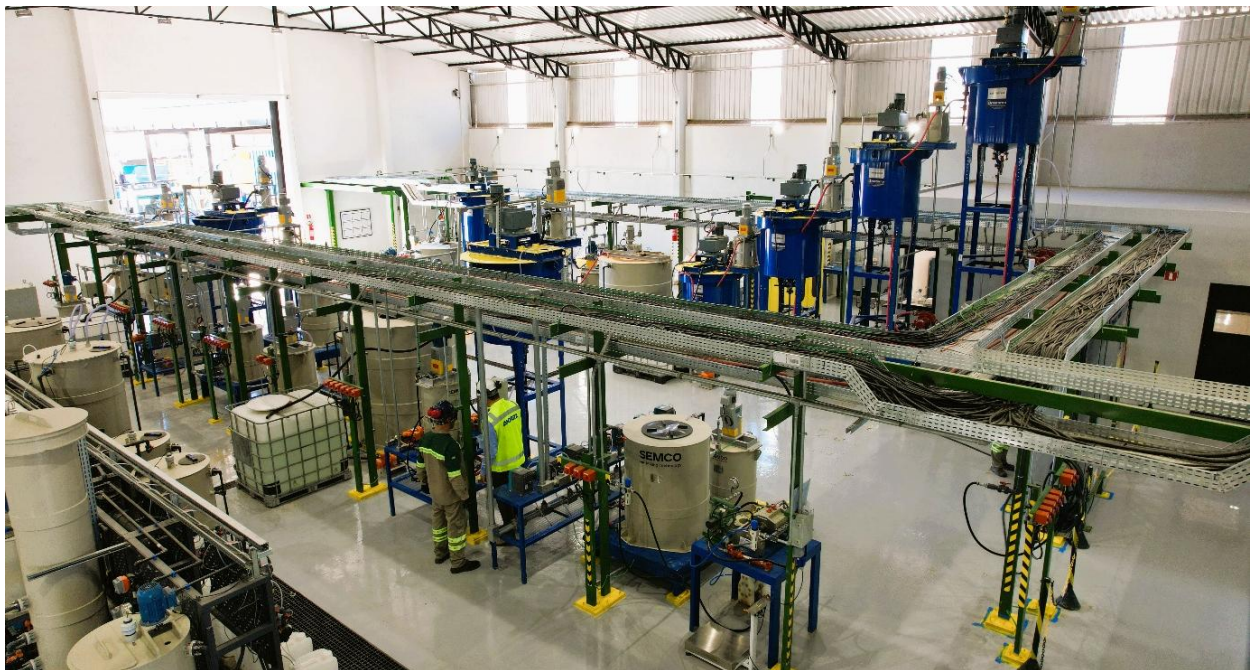
Figure 12: MREC Demonstration Plant is the largest known semi-industrial, continuous operation plant outside China.
