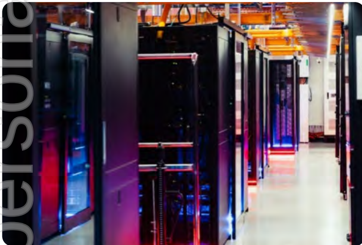
Datacentre220 – our first Express Connect installation
