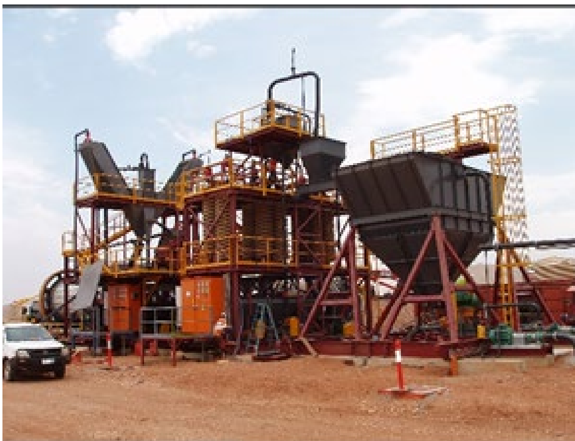
Figure 16: Modular processing plant as previously installed at Tabba Tabba
