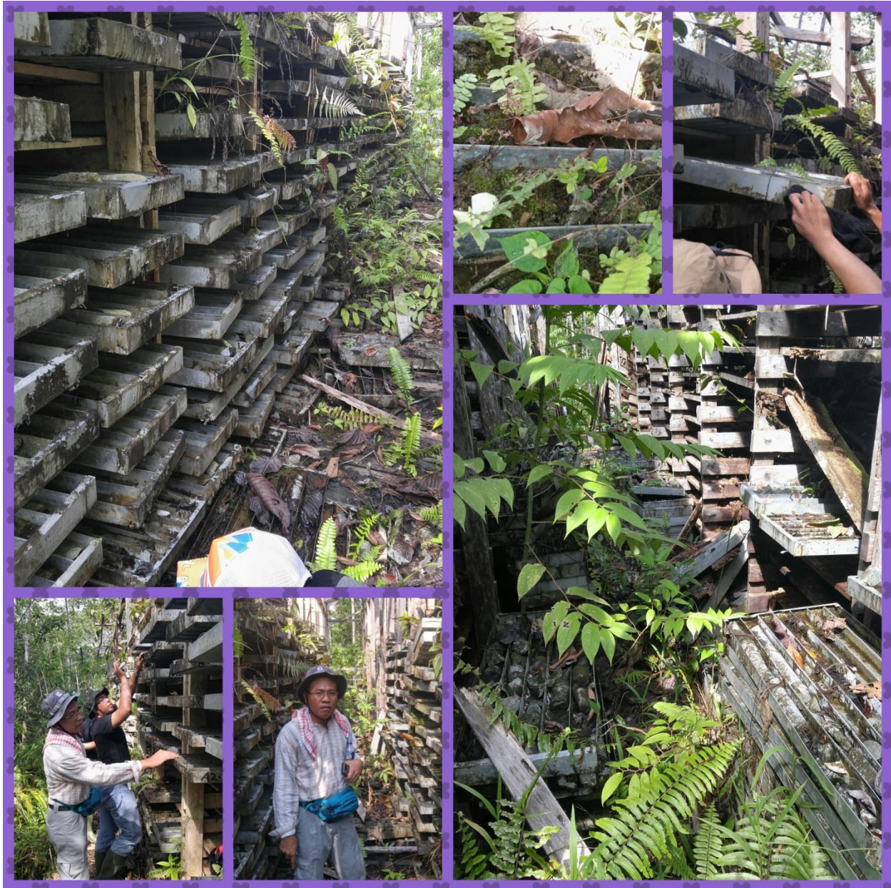
Photo 2. Condition of Tekai Coreshed on 2 November 2016
