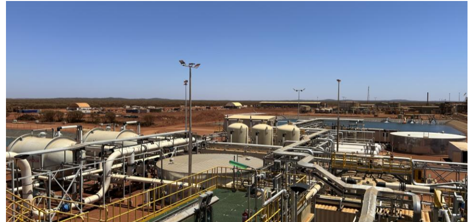
Mt Weld Recycled Water Treatment Plant
