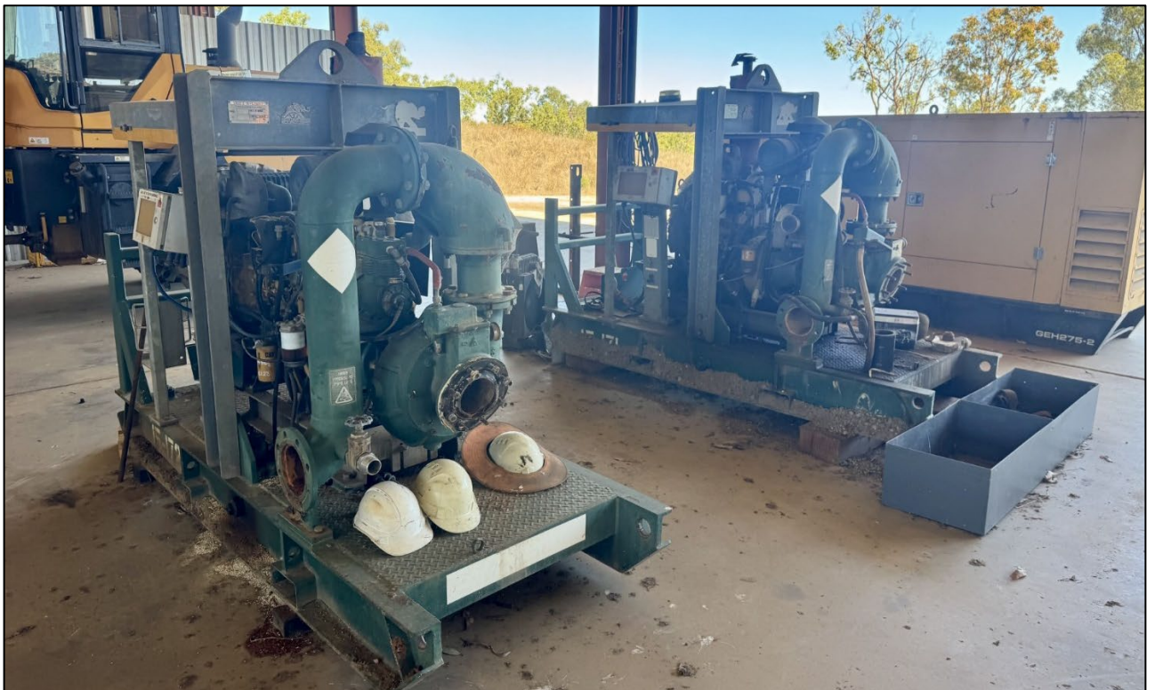
Figure 5: Water pumps in workshop ahead of reconditioning.
