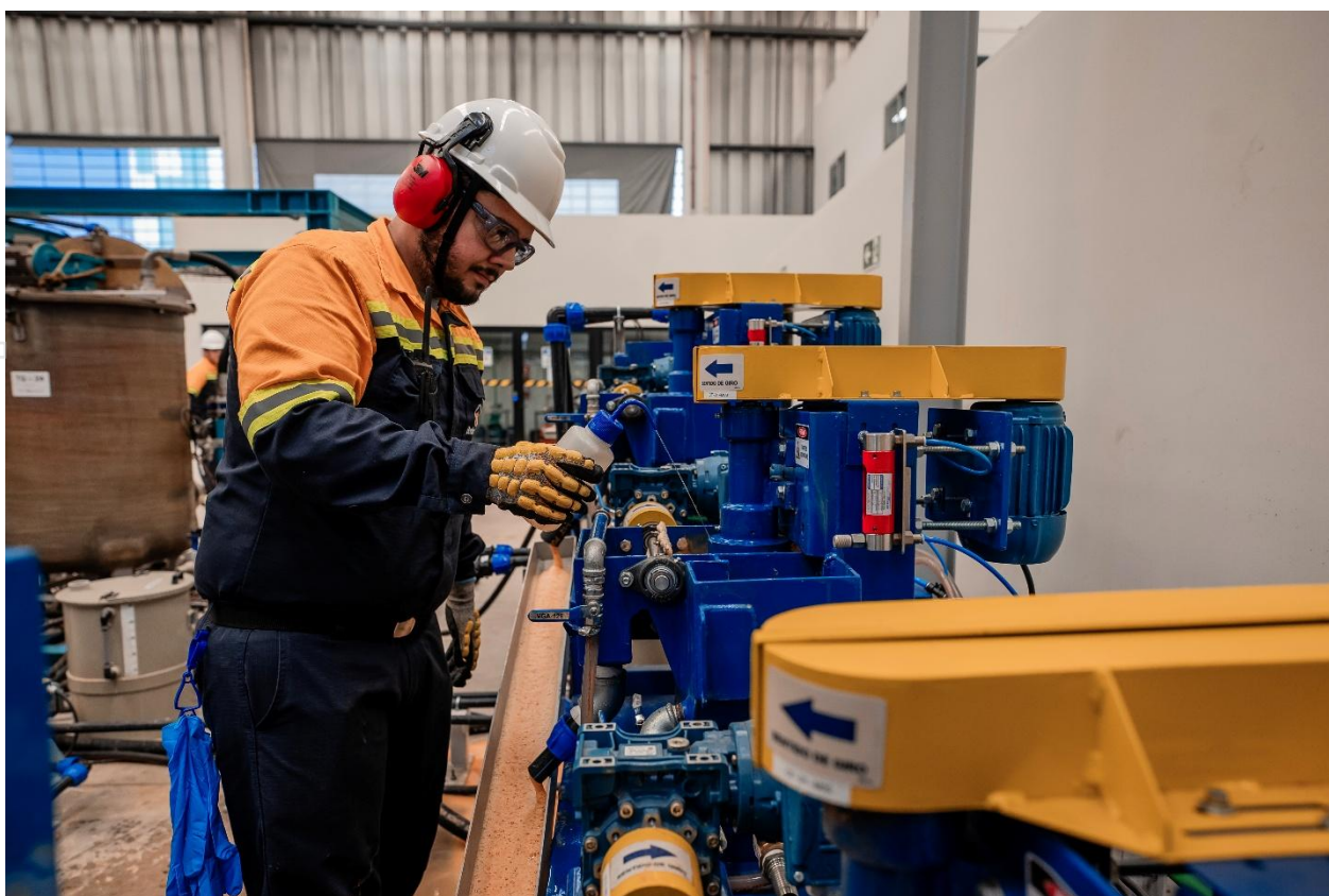
Figure 9: Flotation solution dosing during commissioning.
