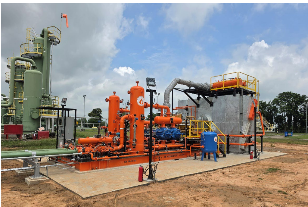
Figure 1: Nam Phong Booster Gas Compressor
