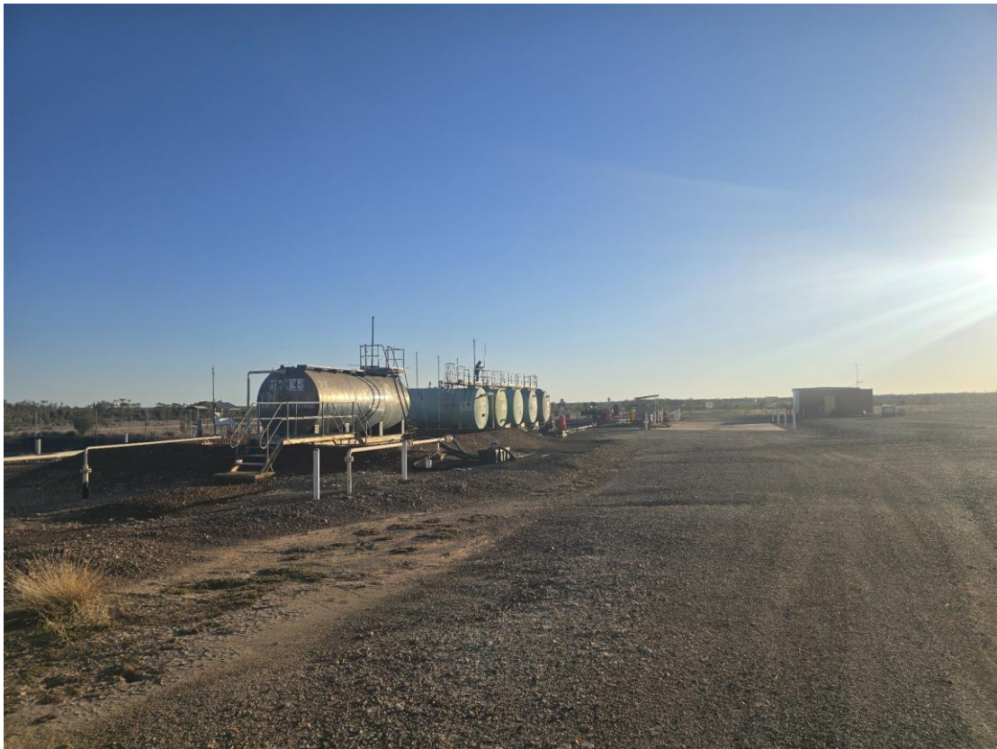
Figure 2 Storage tank levels being dipped to assess timing of next oil lifting
