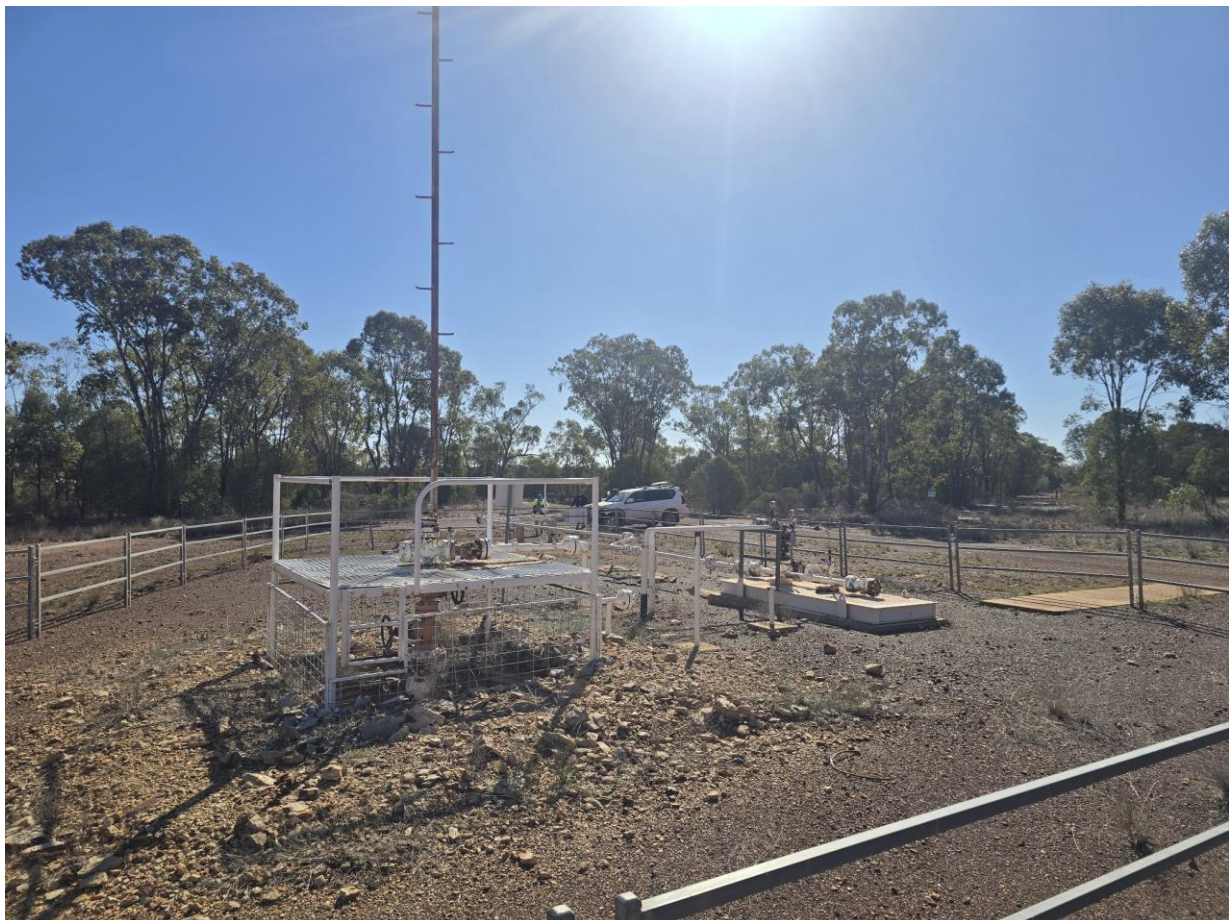
Figure 5 Communications tower at one of the Boxley wells adjacent to the connection to PPL 22 connecting Majo to the line to Silver Springs Plant
