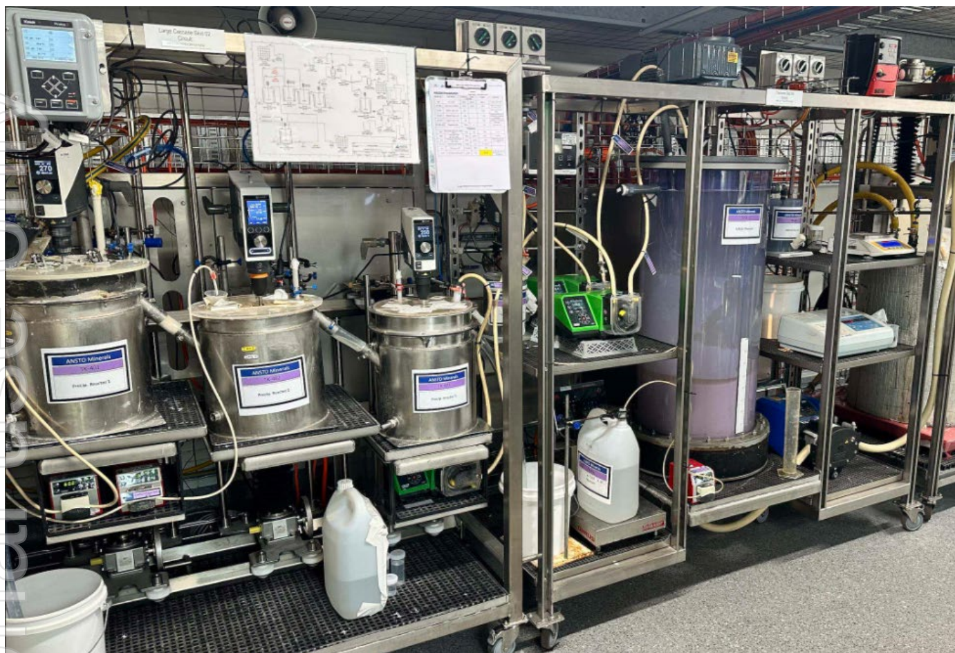
Figure 1: Continuous three-stage precipitation reactor with MREOH accumulating in transparent thickener vessel (RHS)
