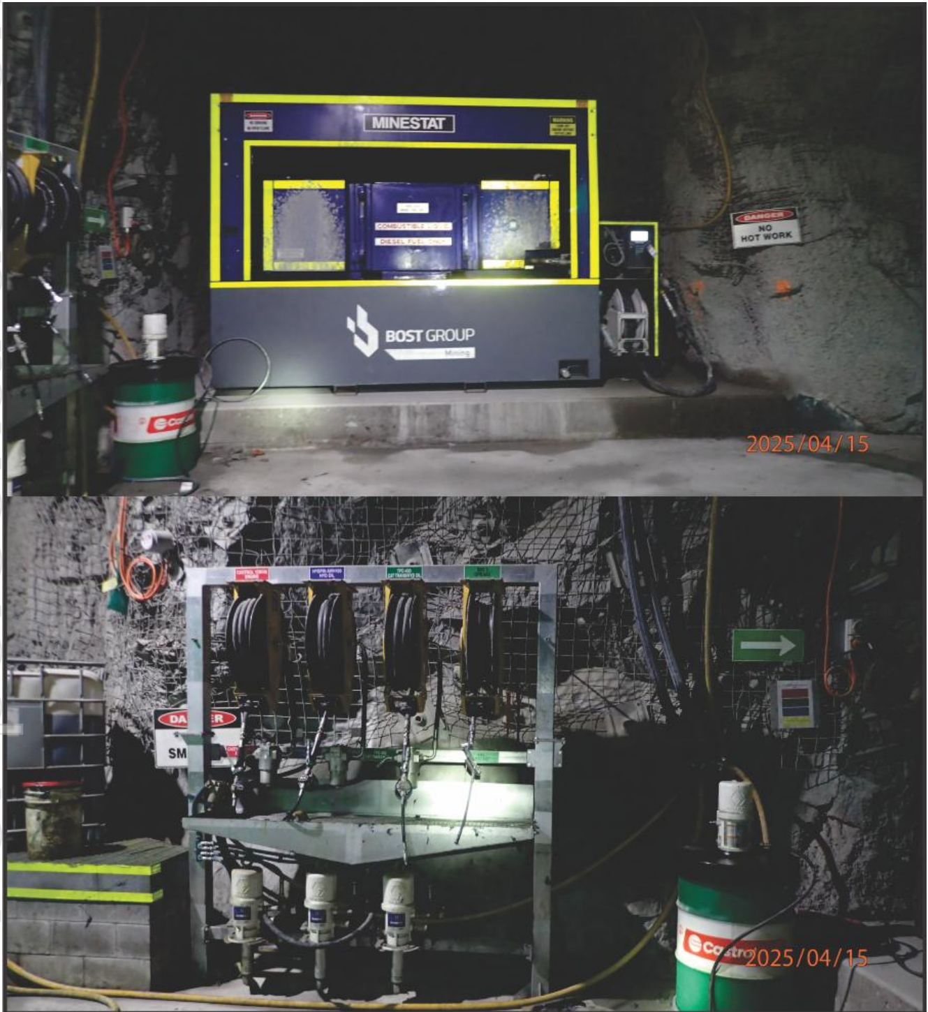
Figure 18-3: Roswell refuelling and lubrication facilities
