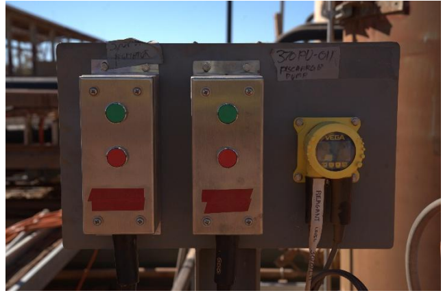
New PLC controls installed
