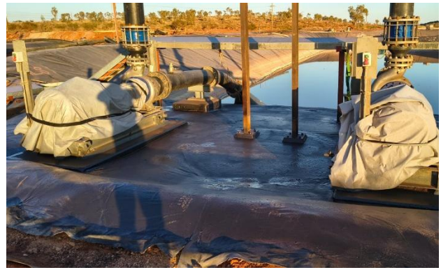
Containment infrastructure around pumps
