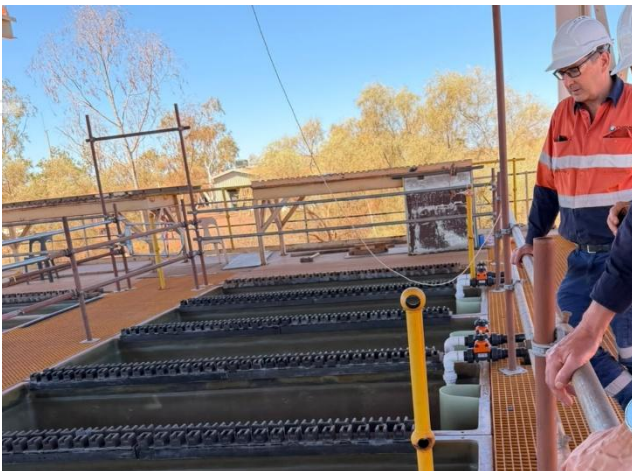
Cell top furniture being installed
