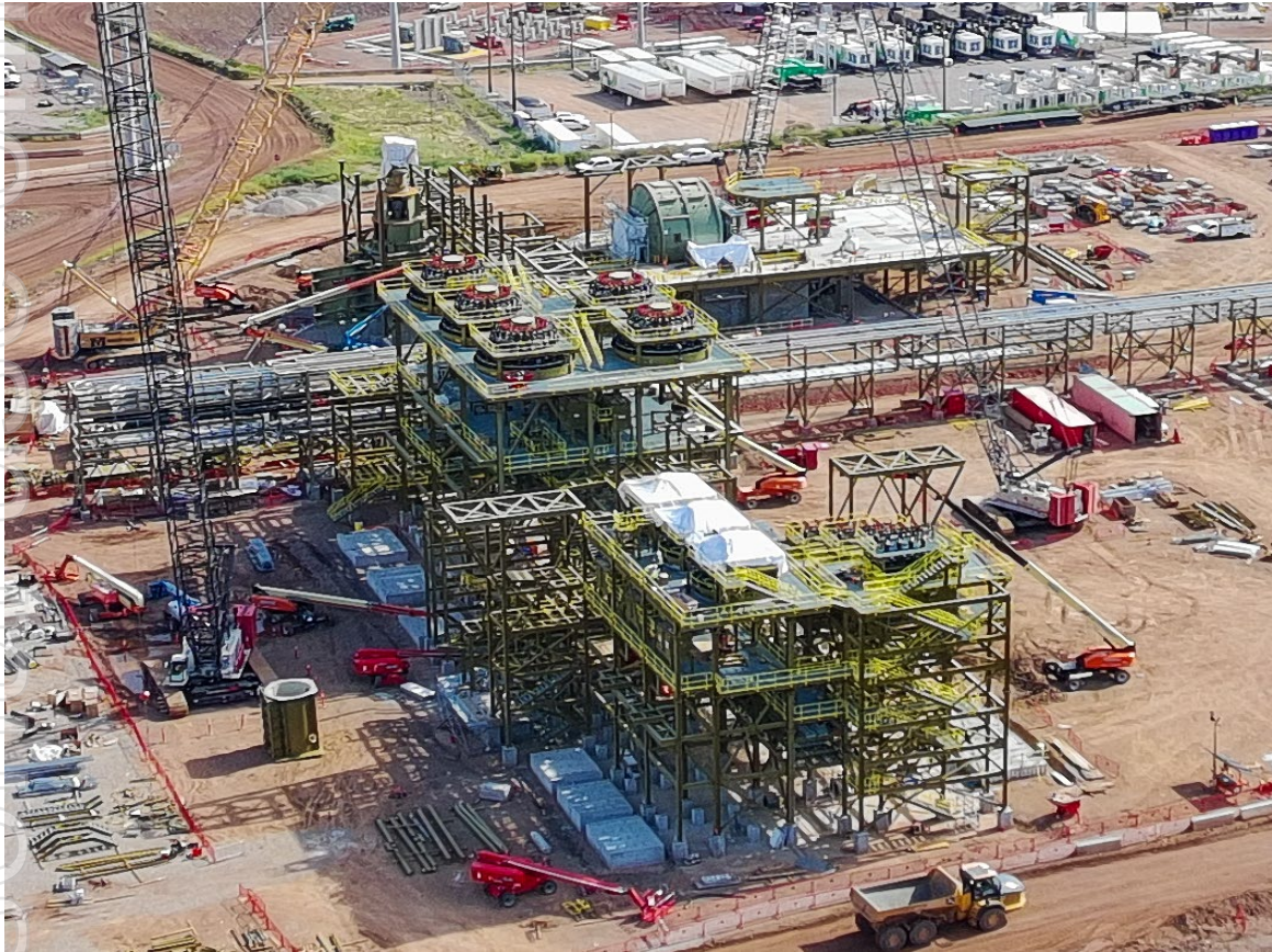
Flotation circuit (looking north)
