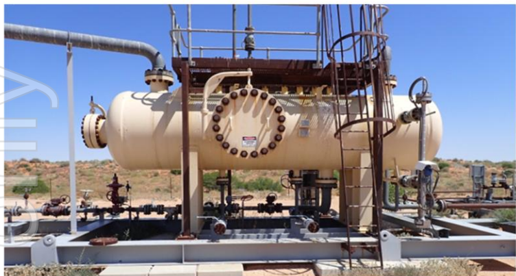
Gas/liquids separator in place at Vanessa facility
